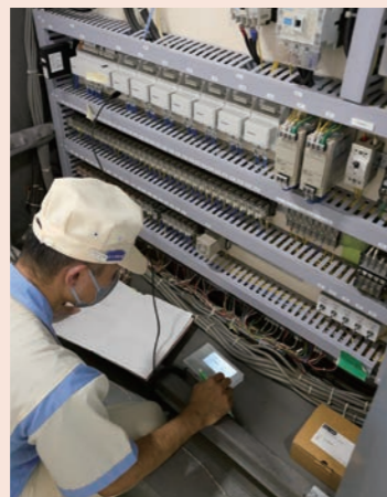
Actual operation and settings of outdoor-air processing unit being checked at factory. Readings are taken daily and temperature and humidity conditions are checked and recorded as part of EMS. Data management helps maintain reductions in the future.
