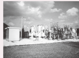
Automated distribution system
